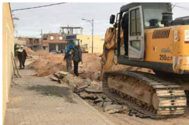
Occasional repair of sidewalks is one way that the Algerian government has attempted to reduce wealth inequality between its provinces.
