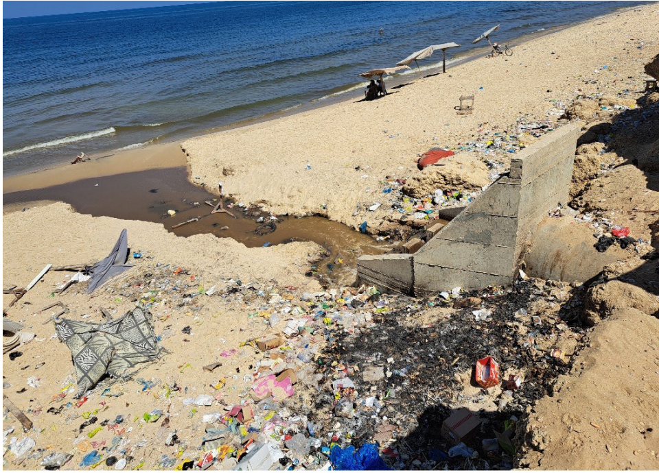
Overflow of raw sewage from a sewage pump station to the Mediterranean Sea due to a deficit of electricity supply, March 2023. Photo by Rebhy El Sheikh
