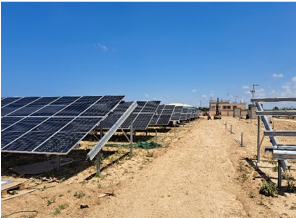
A 7.53 megawatt peak solar energy plant under construction sufficient to operate North Gaza Wastewater Treatment Plant and its Recovery and Reuse Scheme for Irrigation, June 2023. Photo by Rebhy El Sheikh
